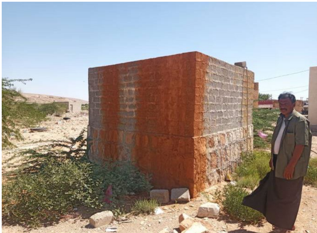
Figure 7: Water tank with iron residues
